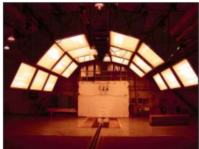
New lighting system in the crash barrier
